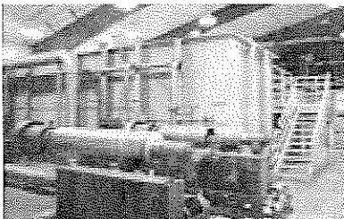
This Amherst, Massachusetts, facility uses ozone technology in conjunction with Trident plants.
