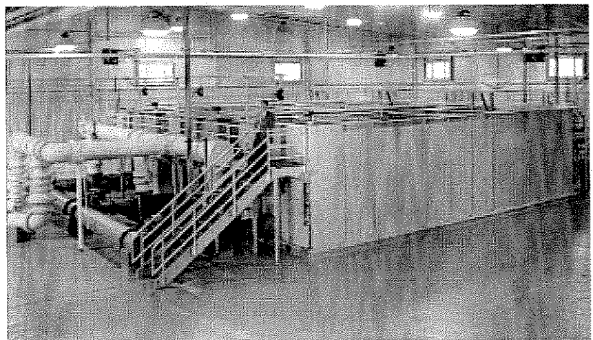
A 6 MGD capacity Trident pre-engineered system is installed in Laconia, New Hampshire.
